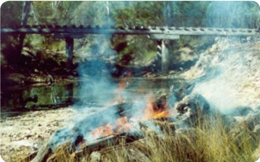
Manual removal and burning of flood debris from around the posts of a historical railroad bridge.
